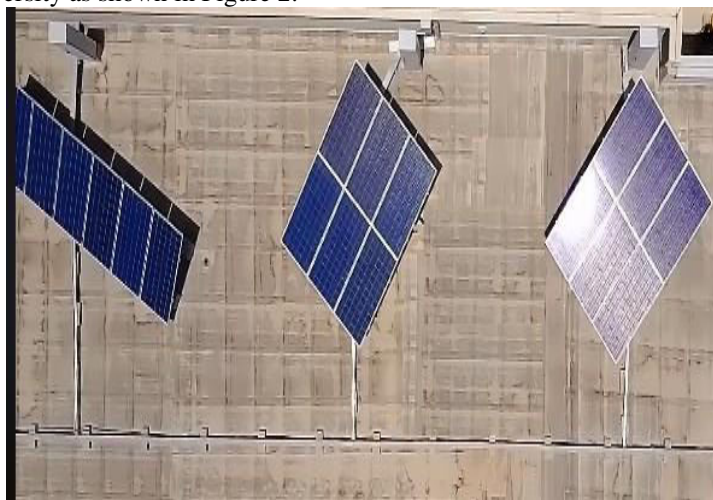
Figure 2 Installations of A Fixed, Single and Dual Axis Solar PV system.
