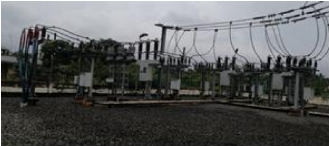
Figure 1: A primary substation
