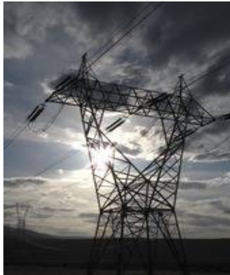
Fig.2.1: 3-phase high-voltage lines in Washington State
