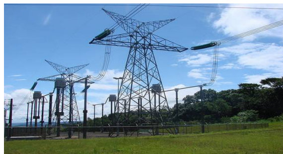
Fig:2.5: HVDC transmission lines
