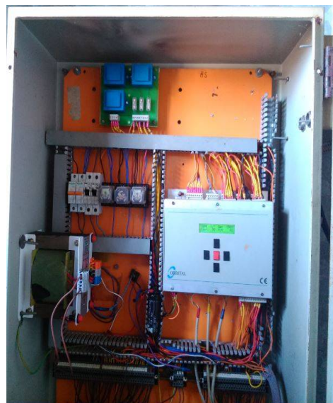
Fig. 3 Control Panel inside tubular tower.
