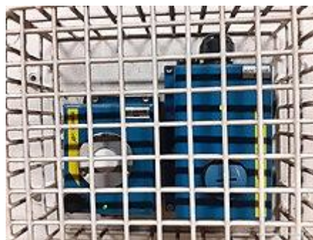
Carbon dioxide and nitrogen dioxide sensors at Birmingham New Street train station.
