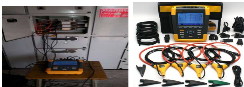
Fig 3 fluke 435 ii series with current and voltage probe and connection with panel
