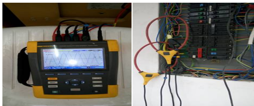
Fig.2. Three phase energy and power quality analyzer ,Fluke 435- II at the field measurement.
