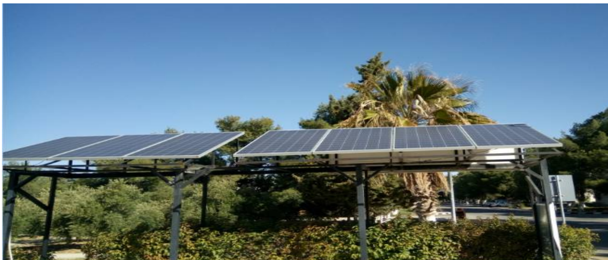
Fig.1. Photo of the PV array under consideration.
