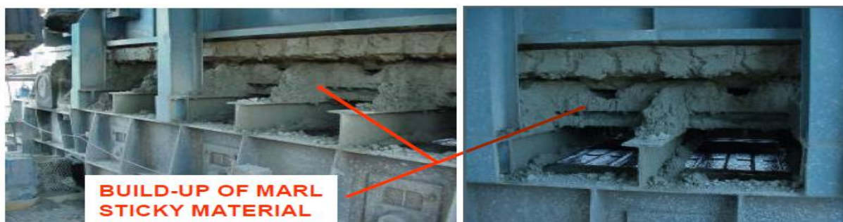
Figure1:Major Problem in the Conveyor System
