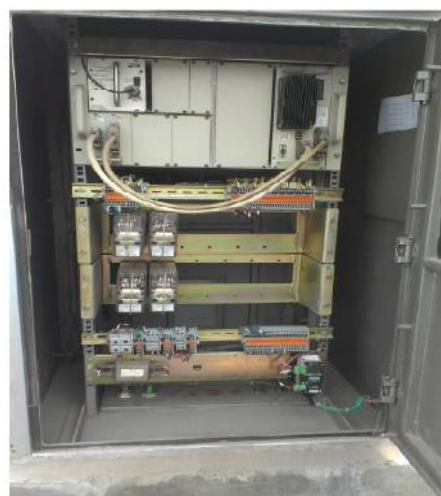
Fig3: LEU cabinet in the field
