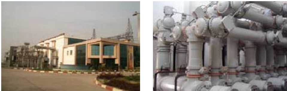
Fig:- 400/220 KV GIS substation at Maharani Bagh , New Delhi
