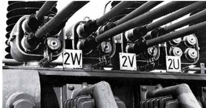
Figure :- cable termination of SF 6 transformer
