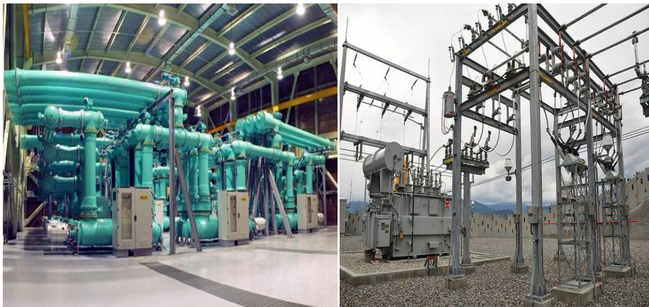
Fig:- Gas insulated substation (GIS) and Air insulated substation (AIS)
