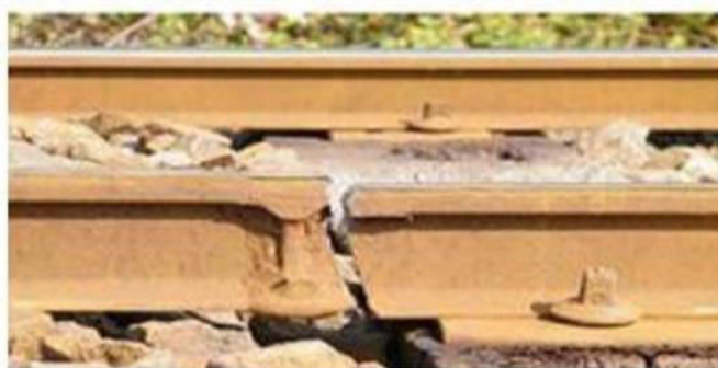
Fig. 1 Crack in Railway Track
