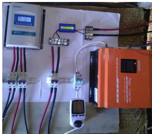
Fig 4. Electric Solar Panel Electricity System
