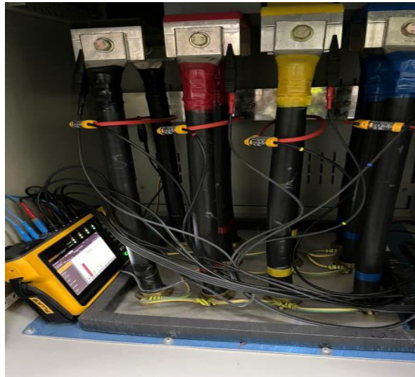
Figure 1. Connection of power quality analyzer device at LV side.
