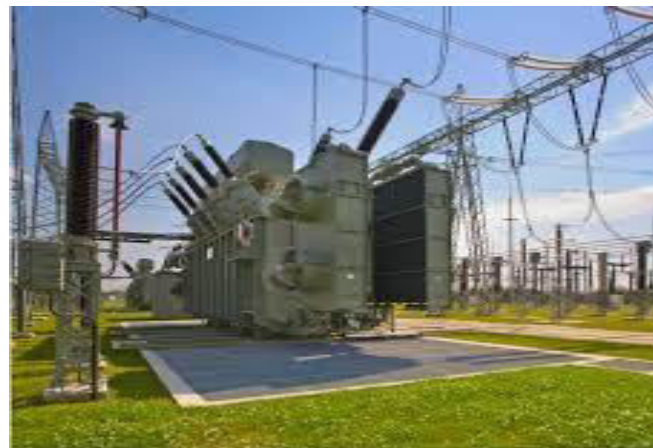
Figure 8Photo of a power transformer
