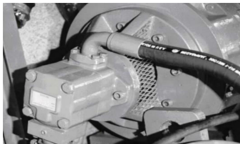
Fig. Close-up of hydraulic pump mounted at the end of the motor shaft.
