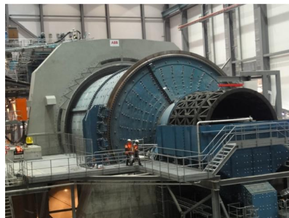
Fig 4- Sag Mill with Gearless motor drive
