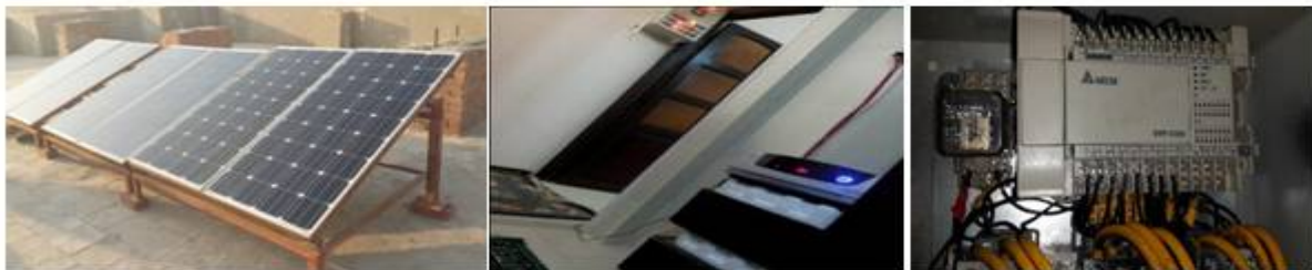
Fig. 7. Implementation of the proposed system. {Solar panels, (ATS, Inverter and Batteries), Delta PLC}
