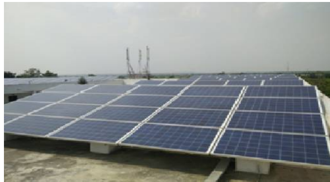
Fig. 1. 100kWp grid connected solar photovoltaic plant installed at BVRIT.
